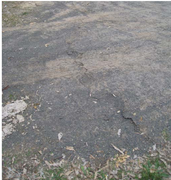
Fig. 4.6 Example of surface compression buckling observed in road pavement (observed in the southern coalfield at a similar depth of cover as the Study Area)
