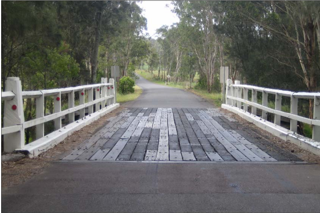
PLATE 1 View of Cony Creek Bridge showing timber deck and guard rail (Item 1)
