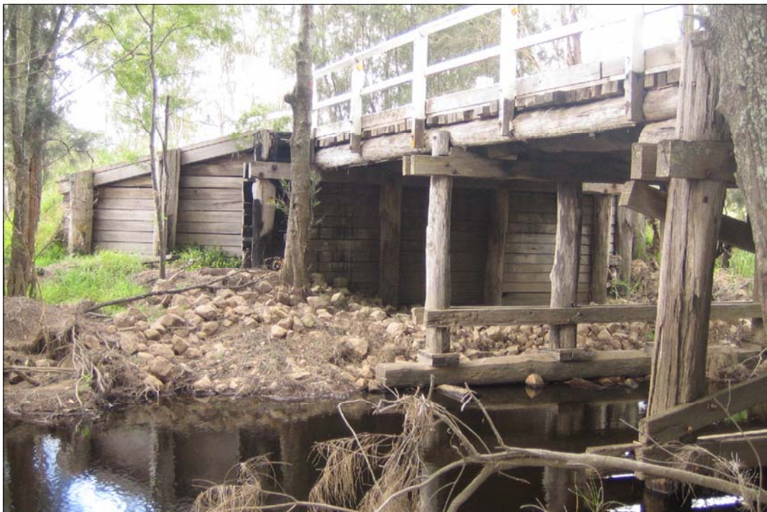
PLATE 2 View of Cony Creek Bridge showing timber piers, trusses and embankment (Item 1)
