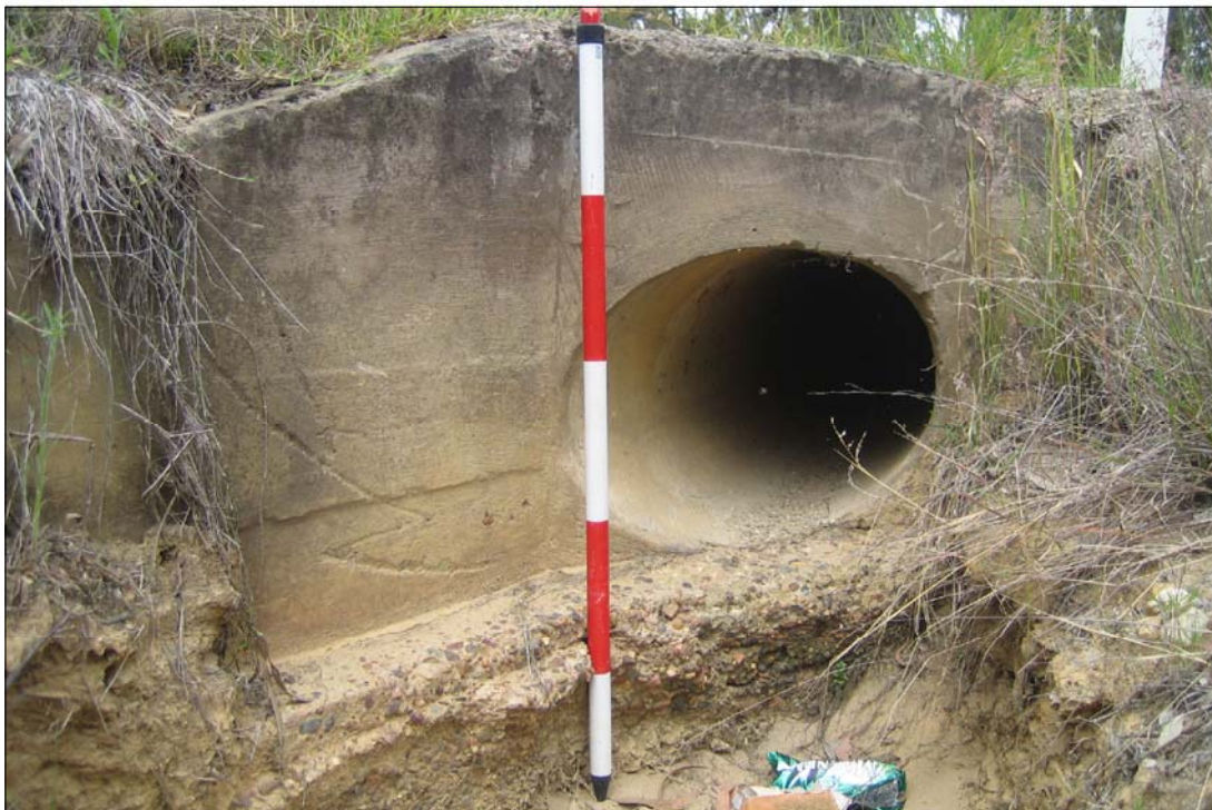
PLATE 8 View of culvert along Quorrobolong Road showing concrete pipe (scale = 1.1m) (Item 7)
