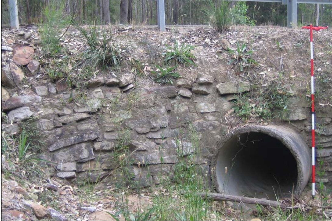
PLATE 7 View of culvert along Quorrobolong Road (Black Creek crossing) showing concrete pipe and sandstone retaining wall (scale = 2m) (Item 5)
