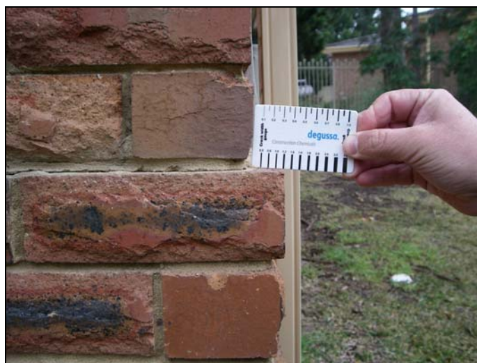
Fig. C.1 Example of slippage on damp proof course
