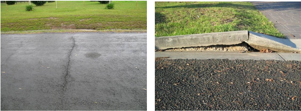
Fig. 6.2 Cracking and Buckling of Kerb at Tahmoor Colliery
