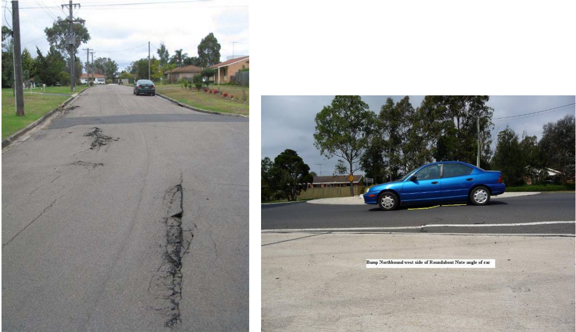
Fig. 6.1 Cracking and Bump at Roundabout at Tahmoor Colliery
