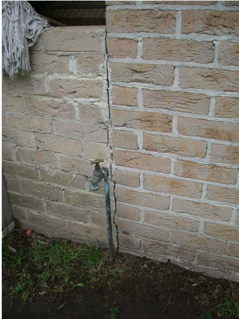
Fig. C.2 Example of crack in mortar only
