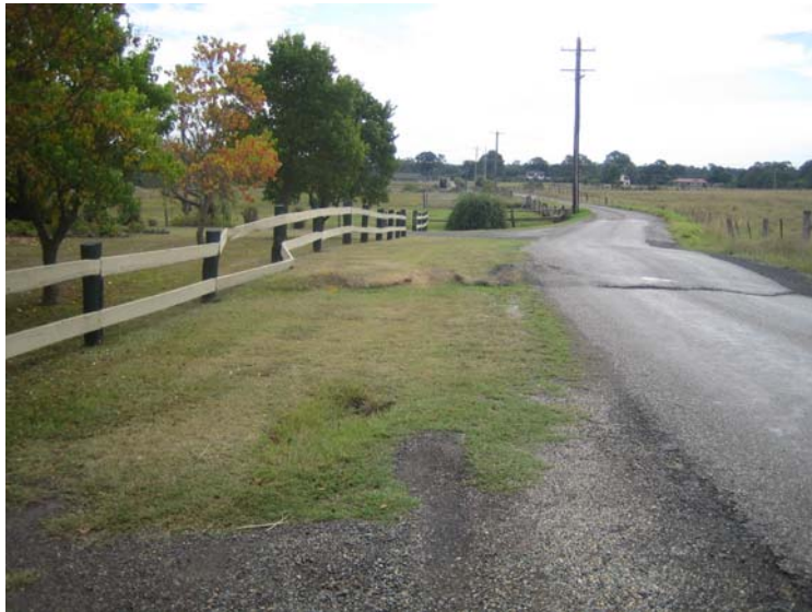
Fig. 4.9 Surface Compression Humping due to Low Angle Thrust Fault (above Appin Longwall 408)
