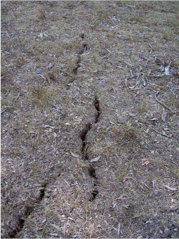
Fig. 4.11 Example of Surface Tensile Cracking in the Natural Ground Surface (Observed in the Southern Coalfield at a Similar Depth of Cover as the Study Area)
