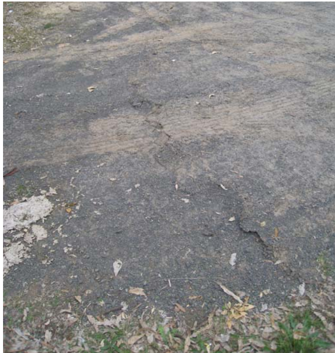
Fig. 5.6 Example of Surface Compression Buckling Observed in Road Pavement
