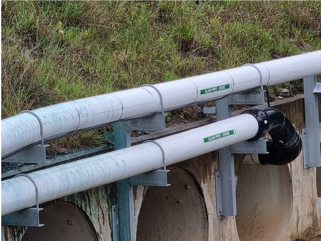
Photograph 13 - Water Supply Pipeline from the Ulan Coal Mine
