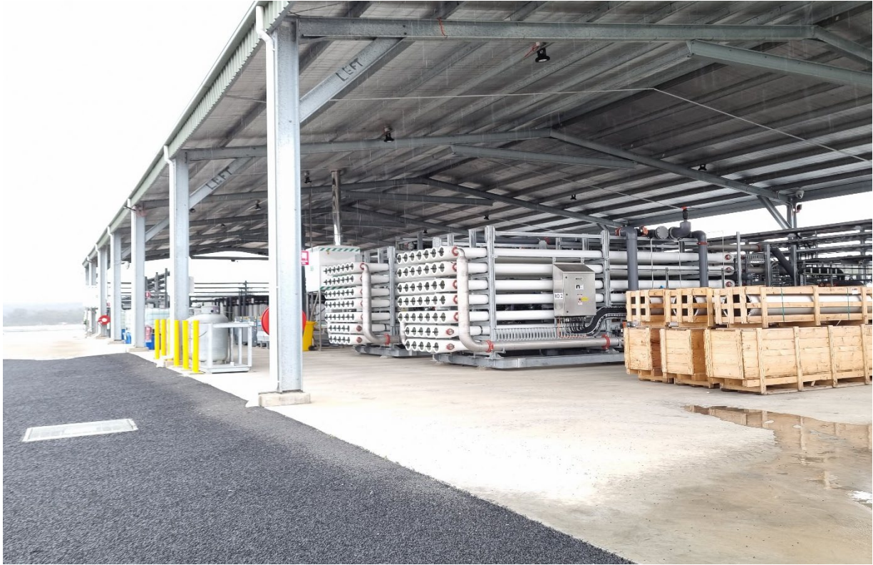
Photograph 5 - Mine Water Treatment Plant
