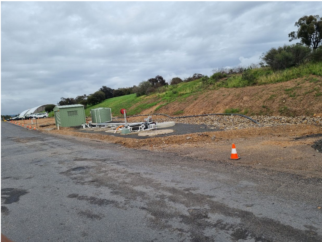
Photograph 16 - Upgraded On-site Sewage Treatment Plant
