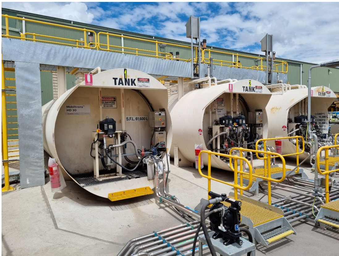
Photograph 14 - Bulk Fuel Storage
