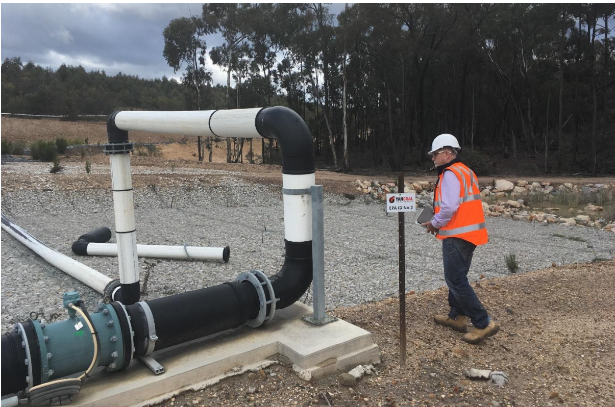
Discharge point with appropriate signage that indicates the EPA point identification number
