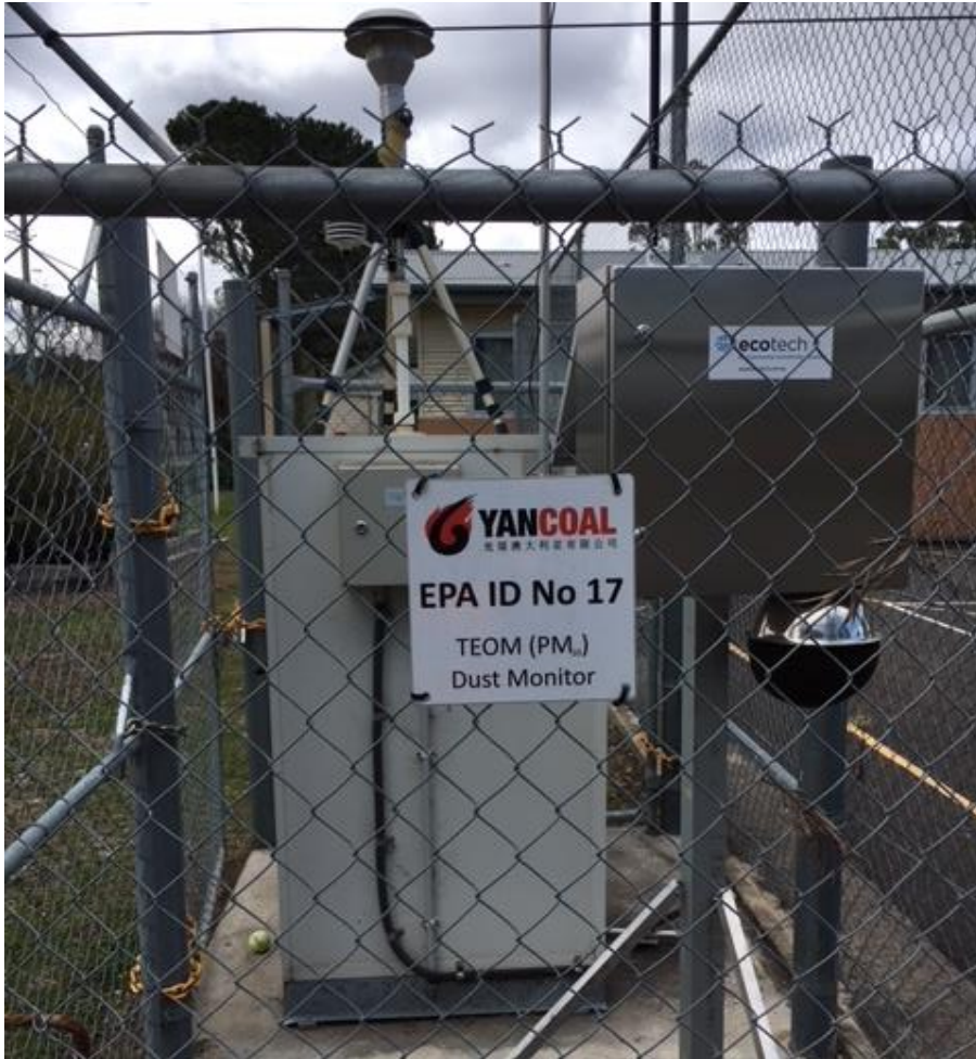
Dust monitor with appropriate signage that indicates the EPA point identification number
