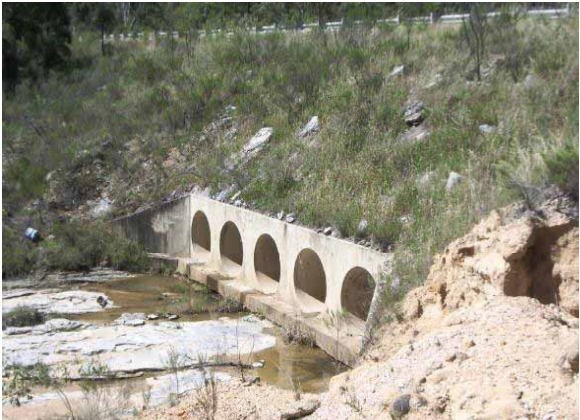
Plate 4 VIEW SHOWING CULVERTS DRAINING RUNOFF FROM BORA CREEK BENEATH THE ULAN – CASSILIS ROAD
