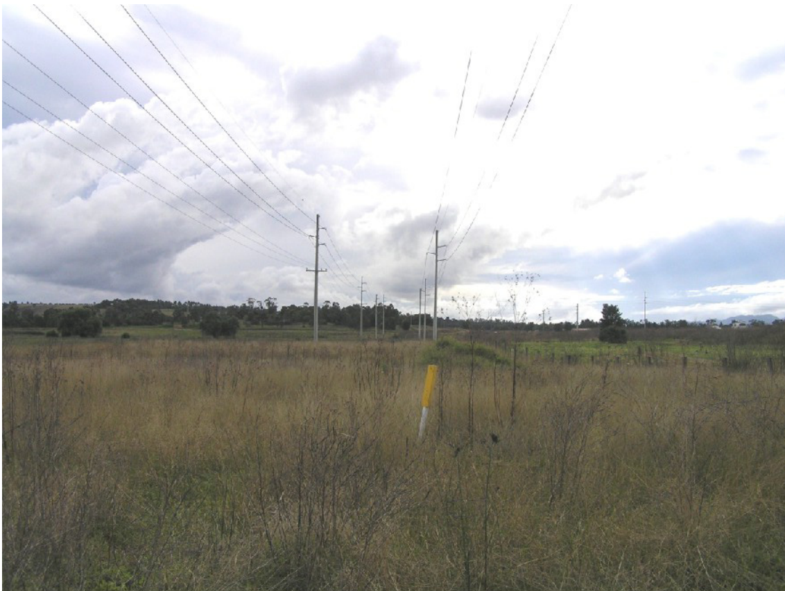
Figure 11: Photograph of Powertel cable and high voltage power lines in New England Highway road reserve.
