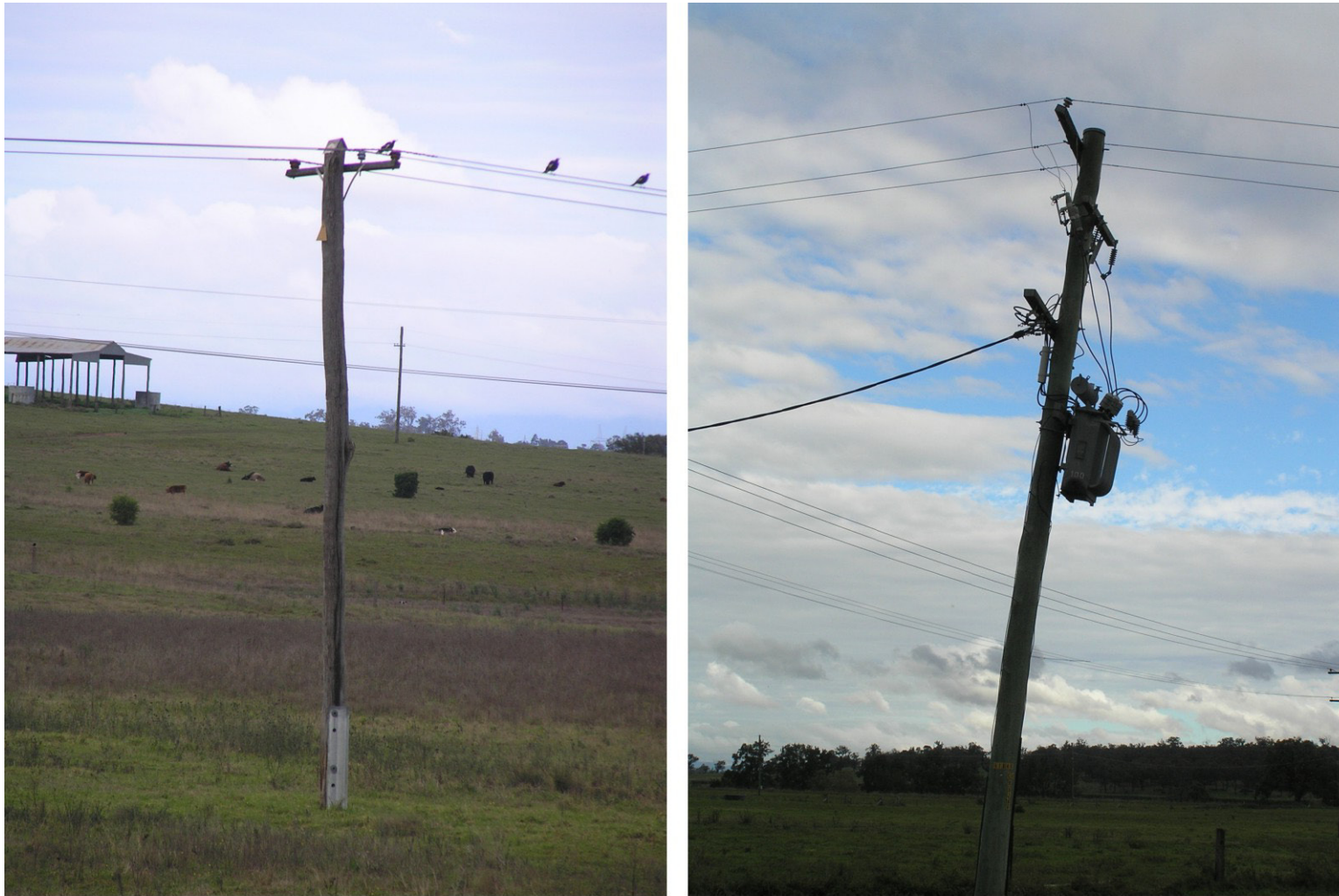
Figure 14: Photographs of single pole structures on local electricity lines.
