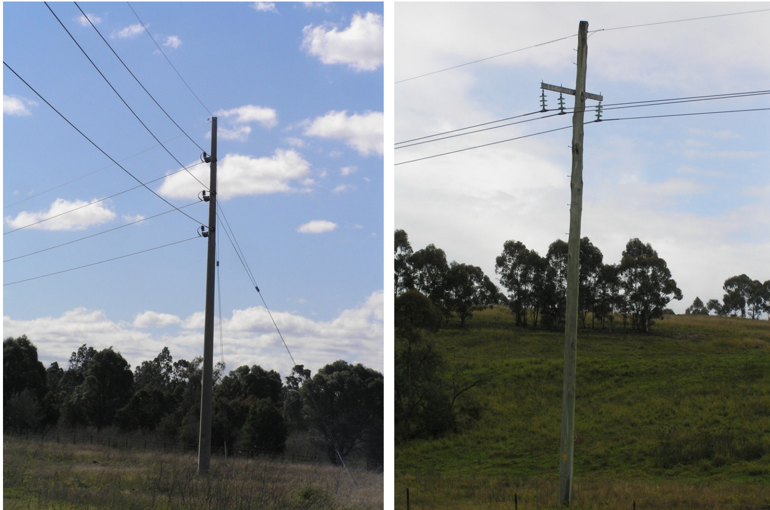
Figure 13: Photographs of single pole structures on 66kV power lines.
