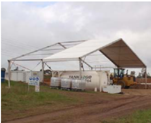
Figure 5 : Photo showing an example of the marquee erected to protect the Raise Bore rig (Source: ACOL)
