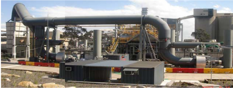
Figure 7: Vocsidizer Installation at West Cliff Colliery (WestVAMP), Australia
