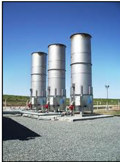
Figure 4: Enclosed flare installation
