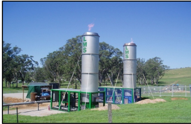
Figure 2: Example of relocatable enclosed flares treating drained goaf gas
