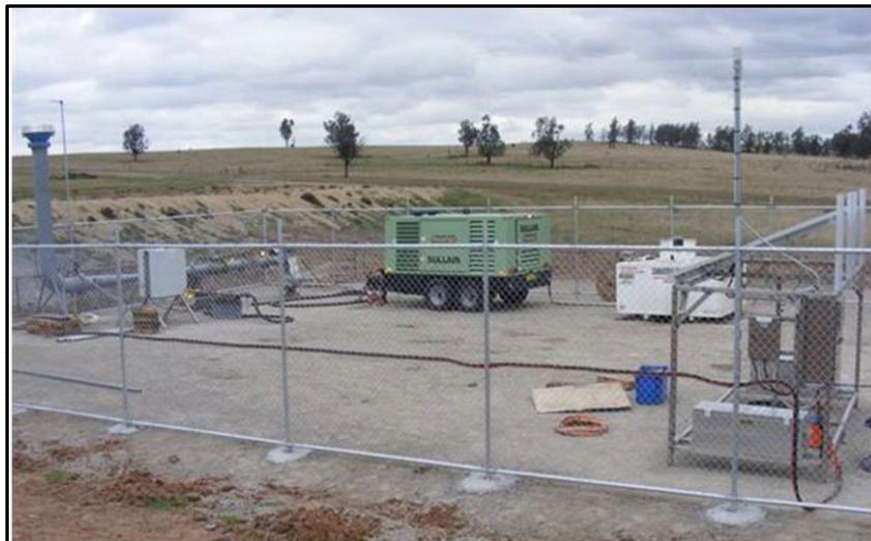
Figure 1: Typical goaf drainage surface equipment layout compound
