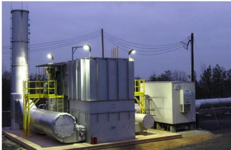
Figure 8: Biothermica – VAMOX Installation
