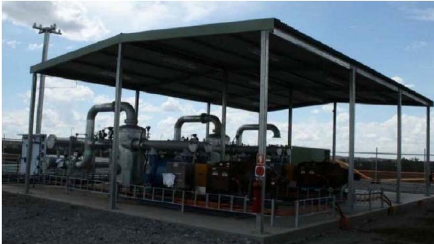
Figure 6: Central gas drainage plant installation
