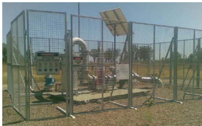
Figure 8: Gas well connection to a gas reticulation pipe network
