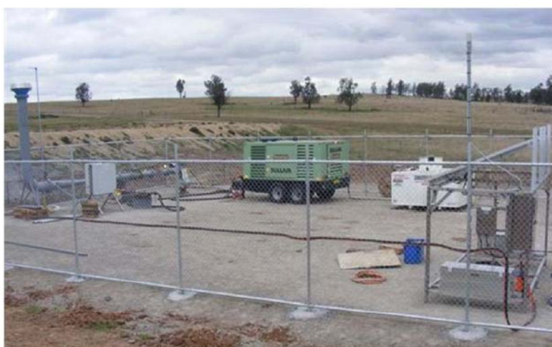
Figure 1: Typical goaf drainage surface equipment layout compound
