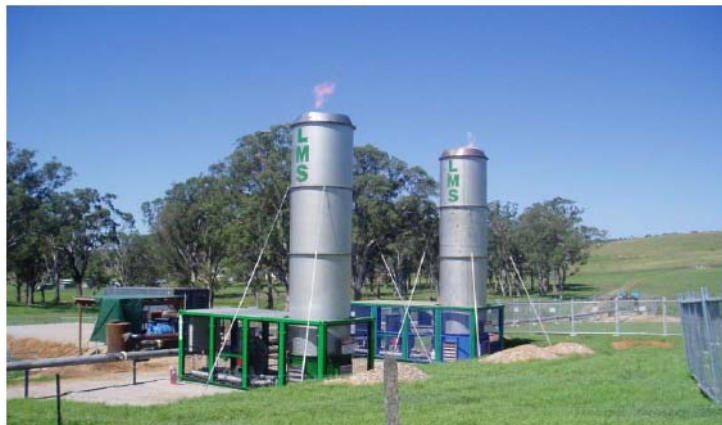
Figure 3: Example of relocatable enclosed flares treating drained goaf gas
