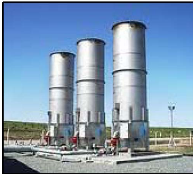
Figure 7: Enclosed flare installation
