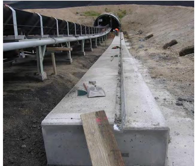
Extension to Product Reclaim Tunnel
