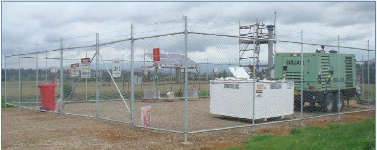
Figure 2. Typical layout of the goaf drainage plant
