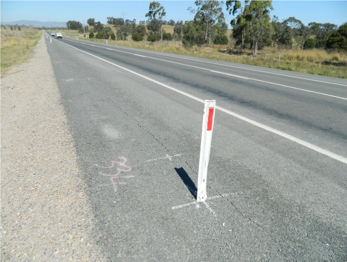
Photograph 11 – Cracking on Lemington Road from mine subsidence
