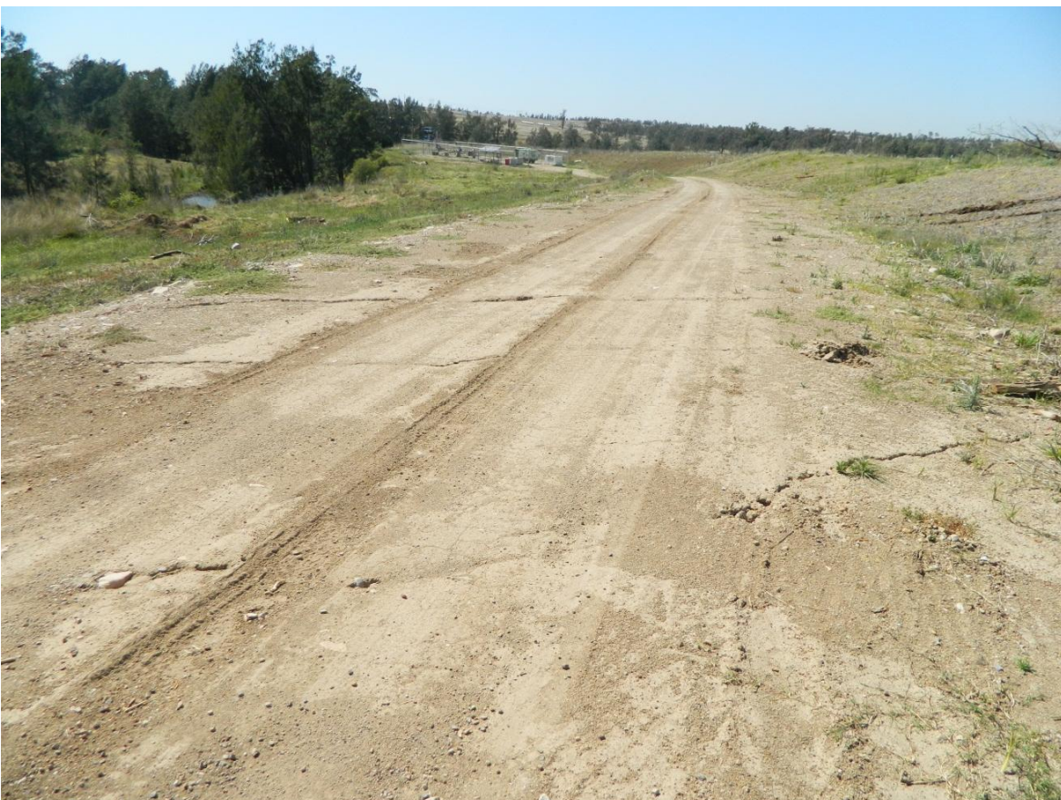
Photograph 12 – Cracking on unsealed road to the south of Lemington Road from subsidence
