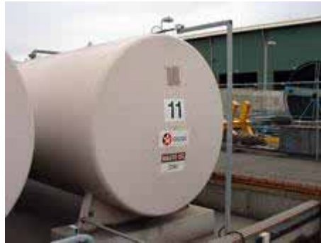
Bulk waste oil storage facility (fully bunded)
