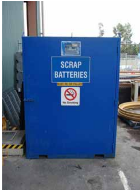
Used batteries are stored inside DG rated Battery storage unit on pallets
