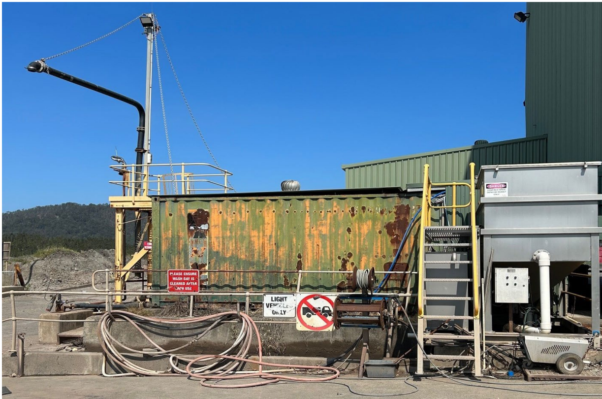
Plate 17 – Oily water separator and storage at pit top
