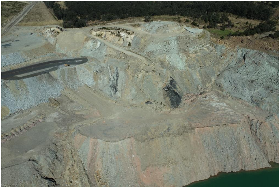
Photo: Rehandle and bulk shaping commencing on the Clareval waste emplacement, July 2021.
