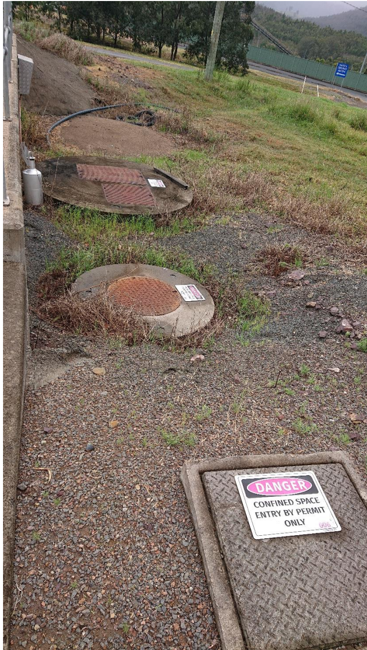
Photo 12 - Oil / water separator
