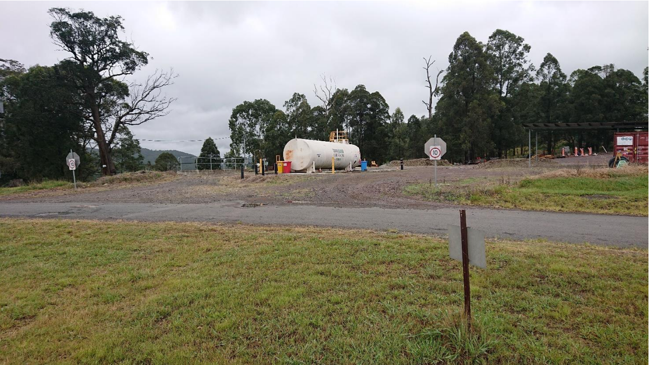
Photo 10 - Bulk Fuel Storage
