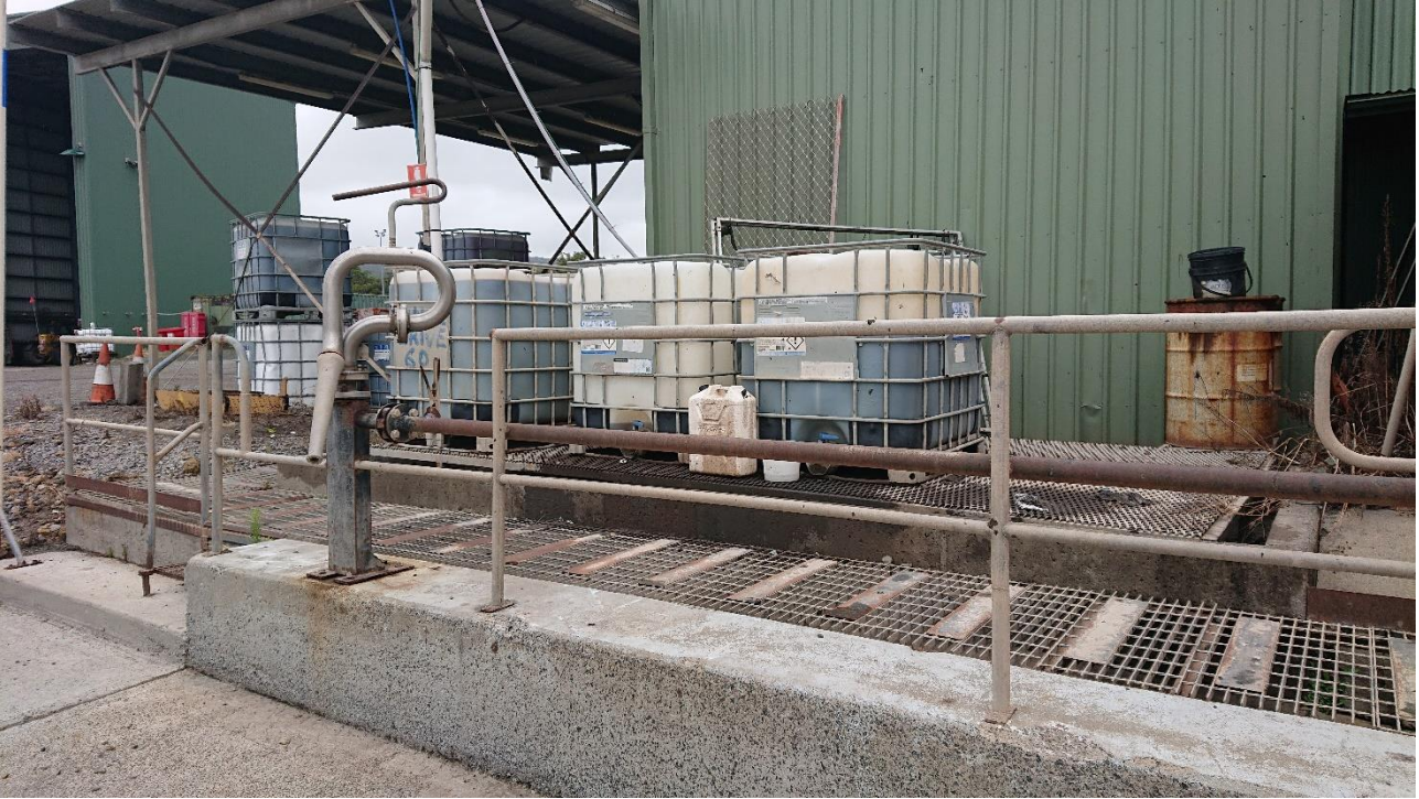
Photo 9 - Waste Oil Storage
