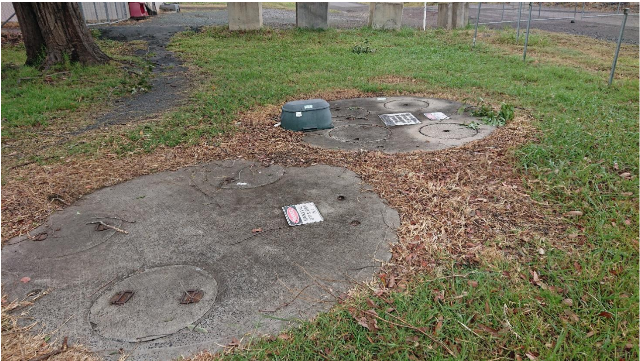
Photo 11 - Wastewater treatment (septic) system
