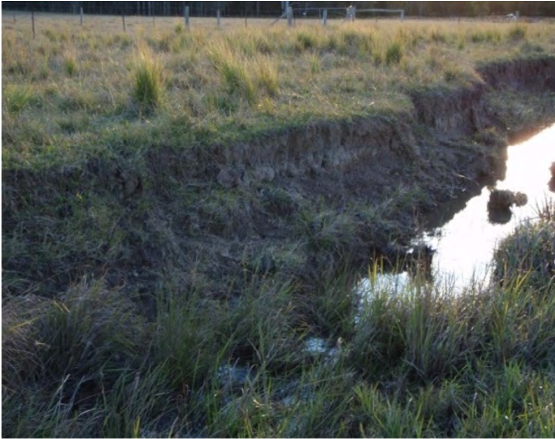
Plate B-2 Avondale Creek North of Roseville West Pit in Area of Channel Excavation
