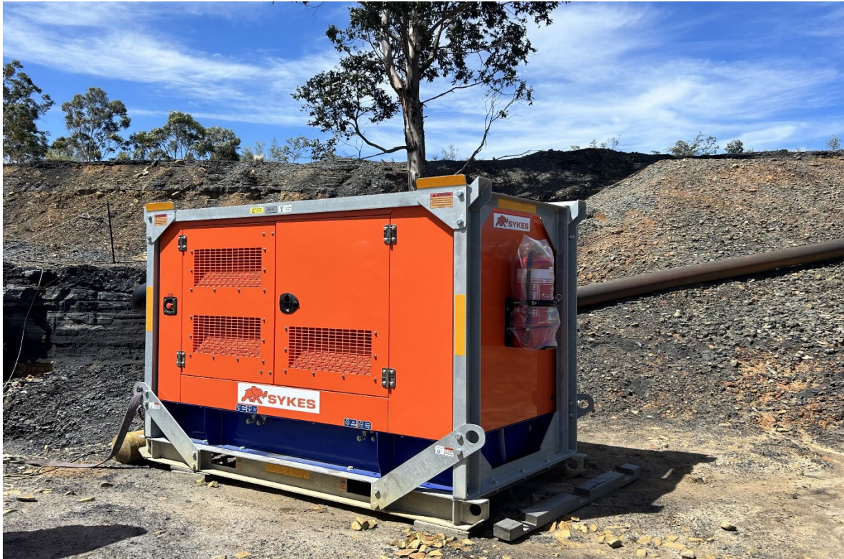
Plate 5 – Containment pump and fire equipment at northwest tailings dam
