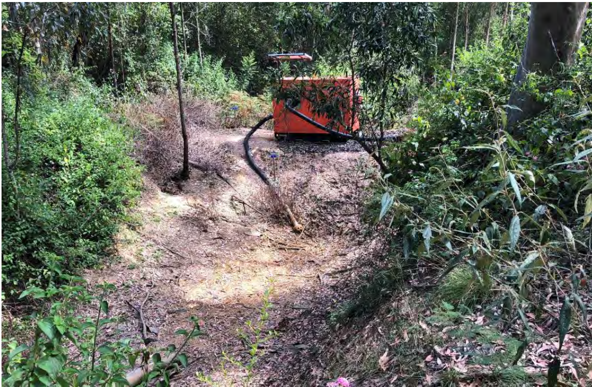
Photo 17 Pump at orange stain clean water drain – consider temporary bunding / spill management
