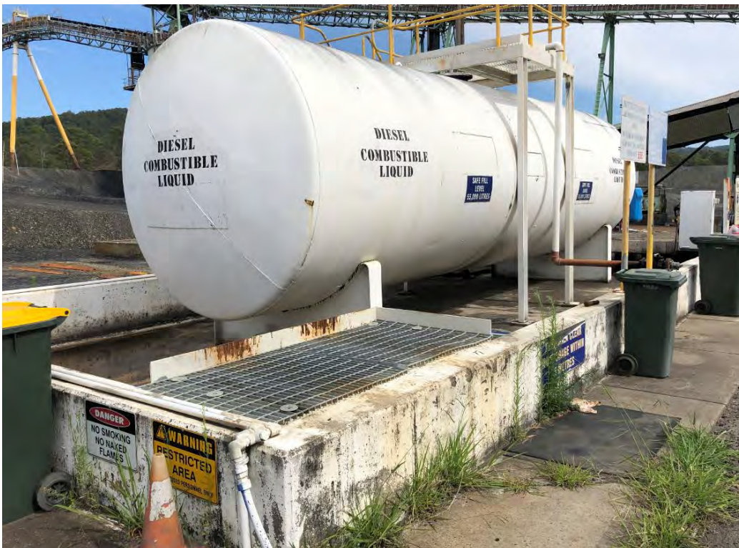
Photo 4 Diesel fuel storage in appropriately bunded areas
