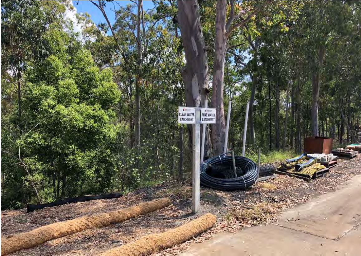
Photo 16 Implementation of Clean/Dirty Water Catchment at Pit Top following previous audit
