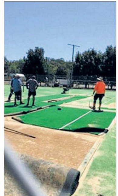
The upgrade involved lifting the carpet and repairing the court surface, shoveling over 30 tonnes of sand off and back on after ground and fence works were completed.
