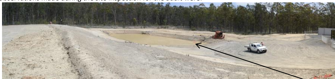
All surface runoff from disturbed areas of the Kitchener SIS drains to major eastern sediment control basin where it may be pumped to Kalingo Dam to retain storage volume in the pond
