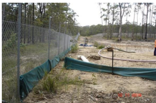
Sediment fence along the boundary of disturbed surface area to reduce the potential for loss of sediment off-site.
