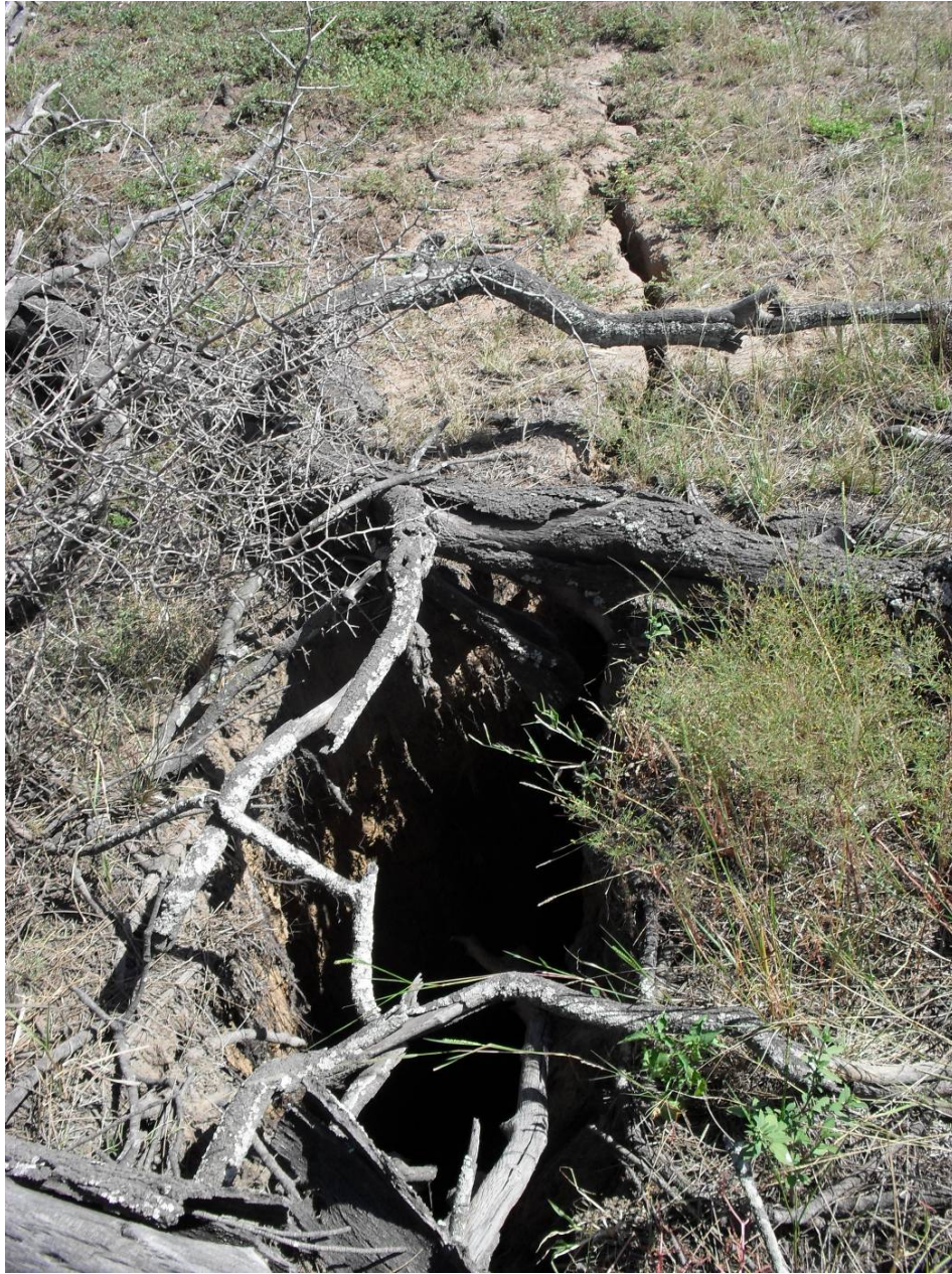
Figure 6: Start line crack in drained dam. This has formed under a tree positioned in the side of the dam wall.
