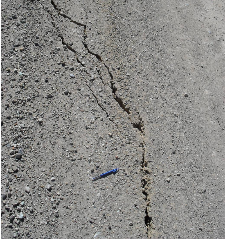
Figure 8: Cracks in the access road which required grading.
