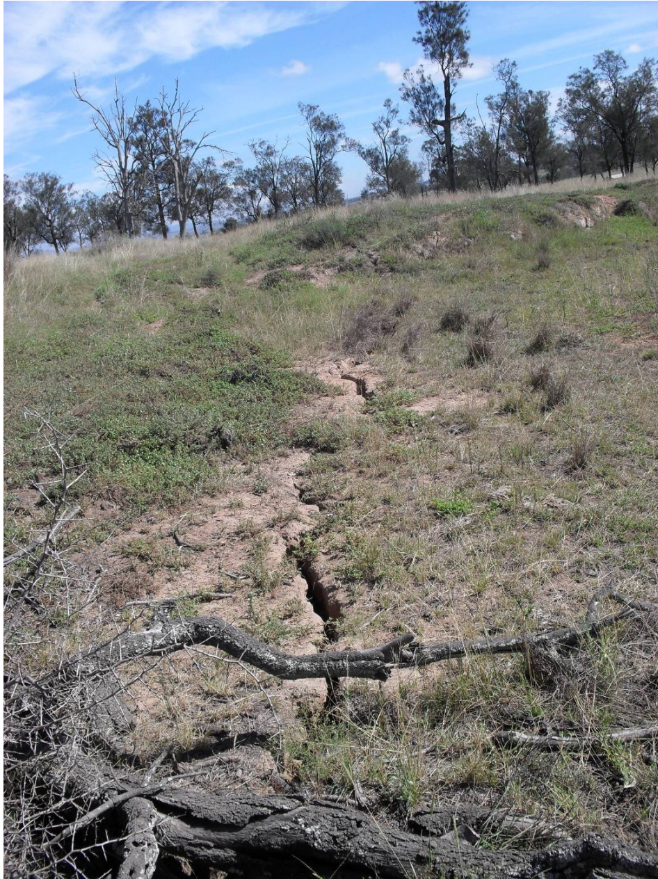
Figure 7: Start line crack continuing up towards dam wall (Background) from under tree. Crack starts from LW4 CL1.
