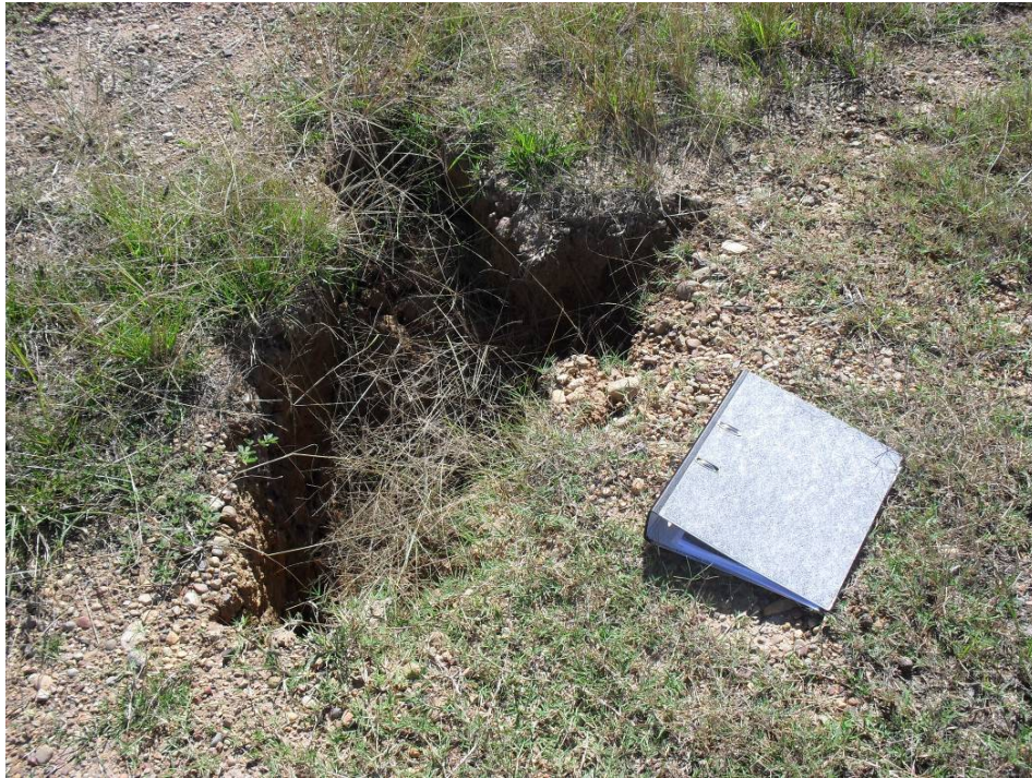
Figure 4: Subsidence in front of Blue House (Chainage 420m)
