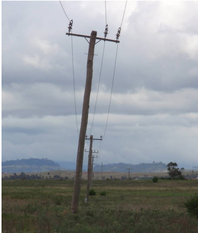
Figure 4: 11kV power line located mid panel in LW7A looking north pre-undermining (05/04/2011). Rollers have been fitted to this line in preparation for undermining.
