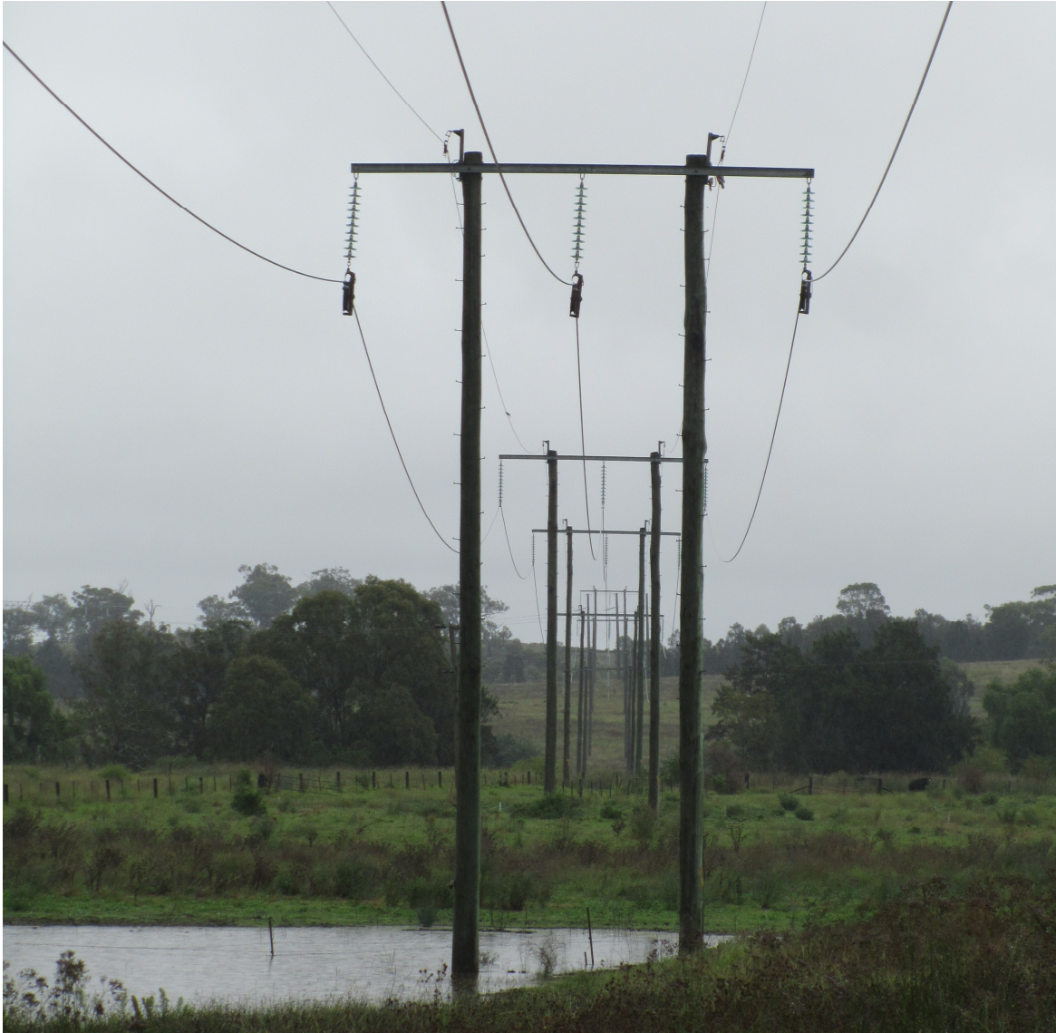
Figure 6: Pole set 11 (foreground) and Pole set 12 (Background) post subsidence.
