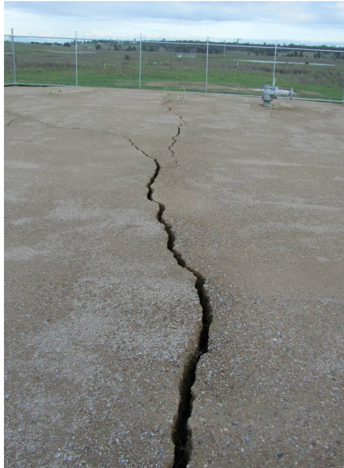
Figure 9: LW7A Gateroad cracking through the compacted pad area at Gas Drainage Plant 5 pre-remediation (16/06/2011).
