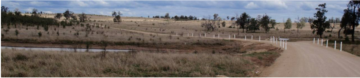
Figure 8: Roadworks completed on the dirt access road to install suitable drainage for the Longwall 3 ponding.
