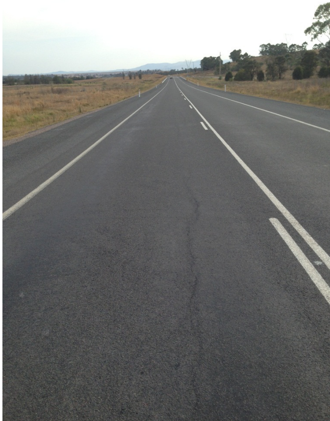
Figure 4 Minor cracking observed on Lemington Road (Looking South)
