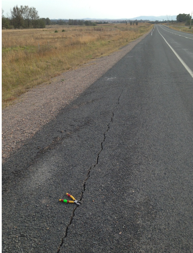
Figure 3 Minor cracking observed alongside Lemington Road (Looking South)
