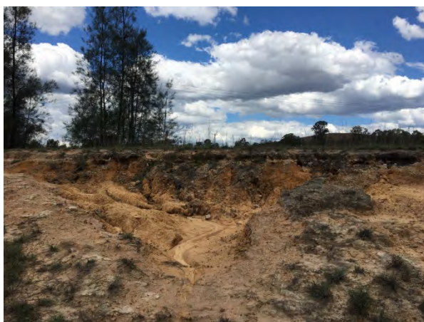
Plate 9 Erosion (top of right bank)
