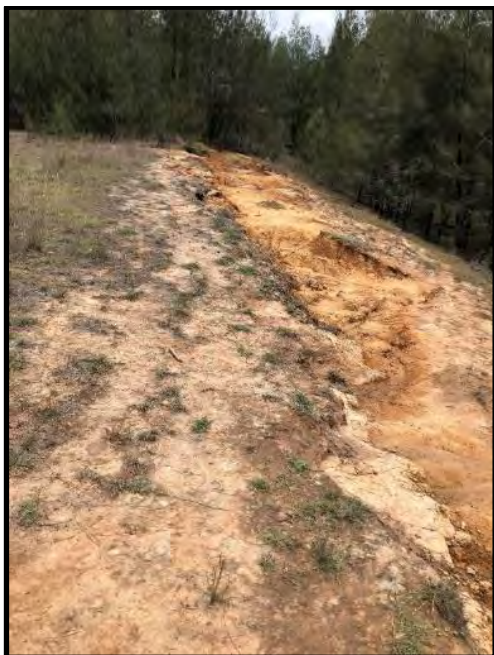
Erosion at MTW-632
