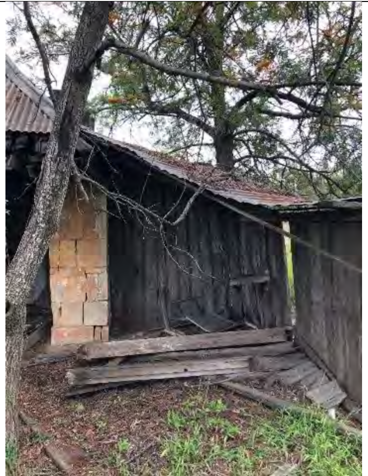
South-east corner: shows removal of vertical slabs from southern wall and further collapse of roof.
