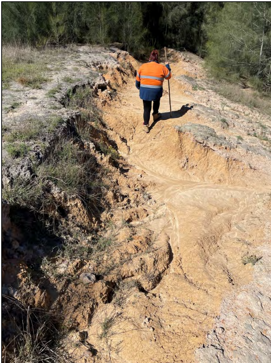
Severe erosion at MTW-632
