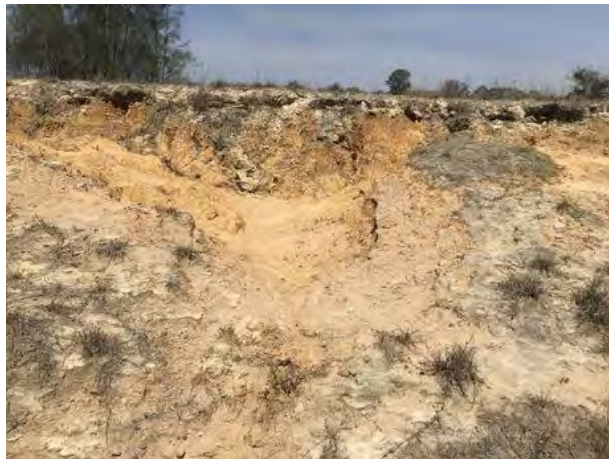
Plate 9 Erosion (top of right bank)
