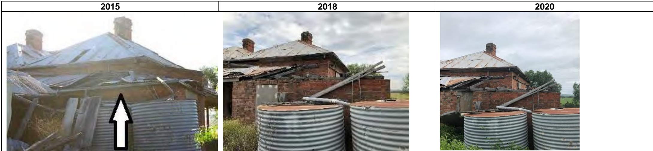
View of rear of building (focus on skillion roof) 2015-8: skillion roof and rafters have collapsed 2018-20: no discernible change
