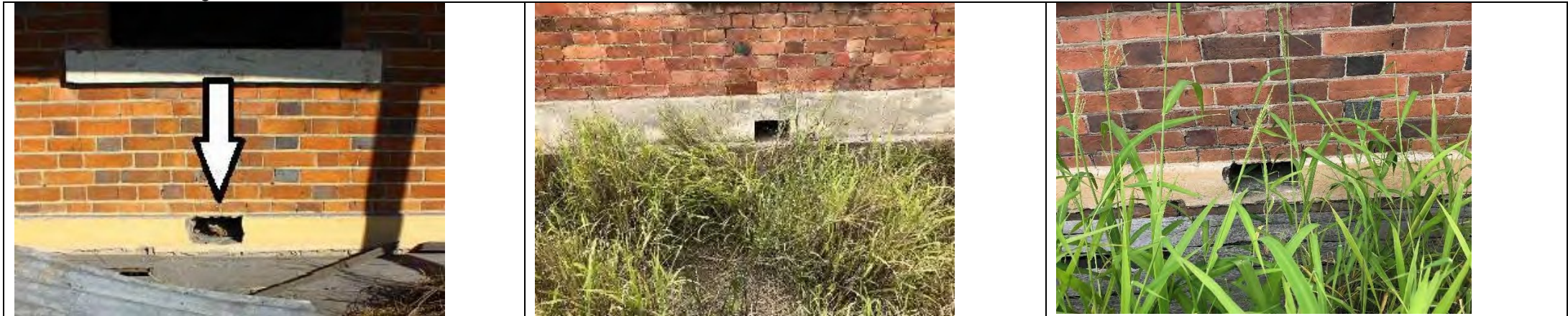
View of ventilation grilles
