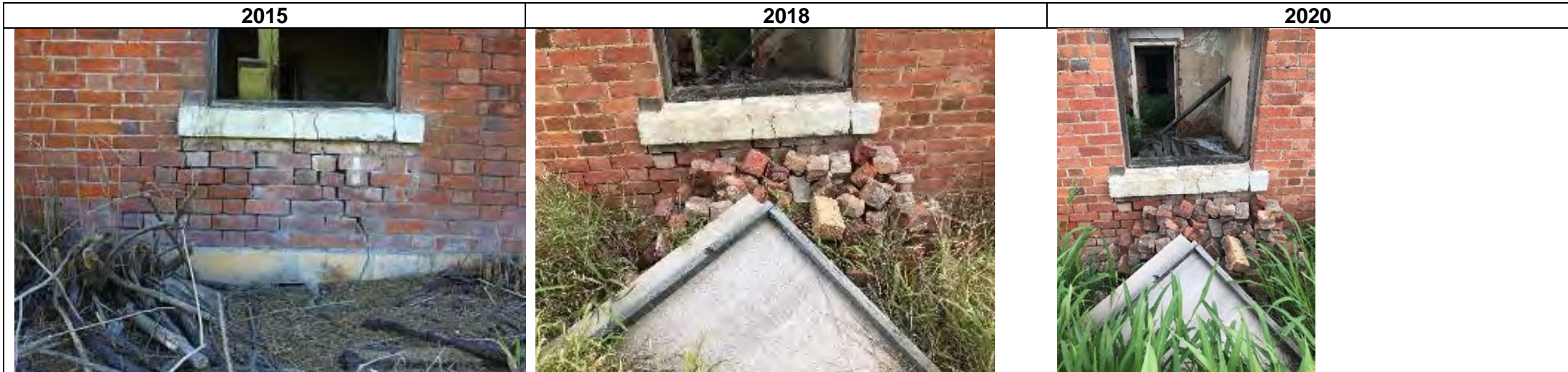
View of north-east corner of building (focus wall below window) 2015-8: bricks from roof above stacked in front of required repointing, window sheeting removed 2018-20: no discernible change
