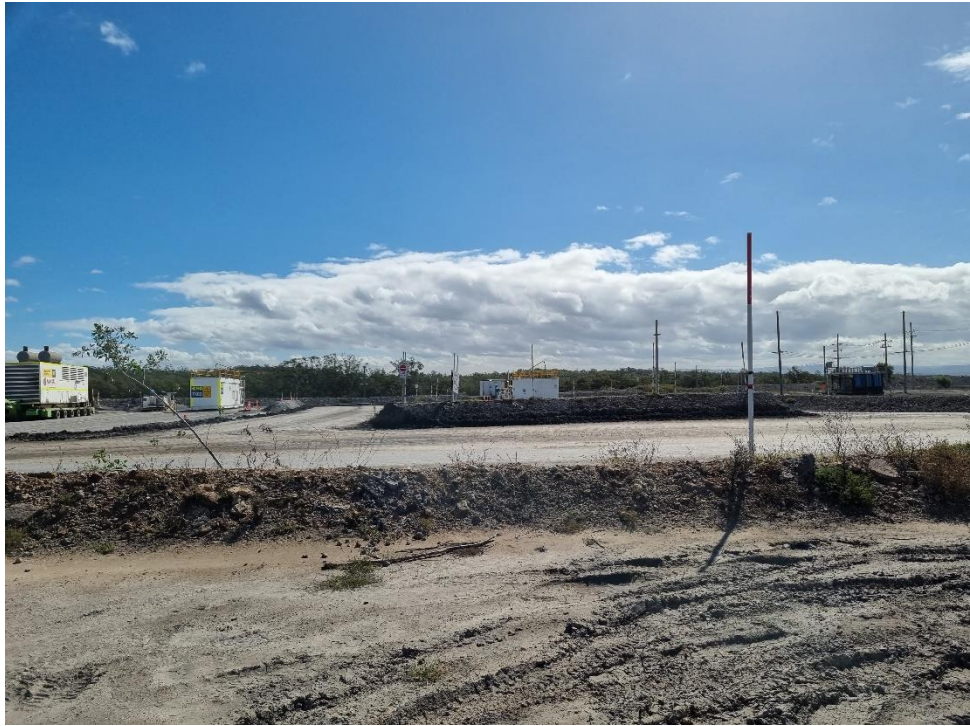
Photograph 9 - Self Bunded Fuel Tank and Generator (Warkworth)
