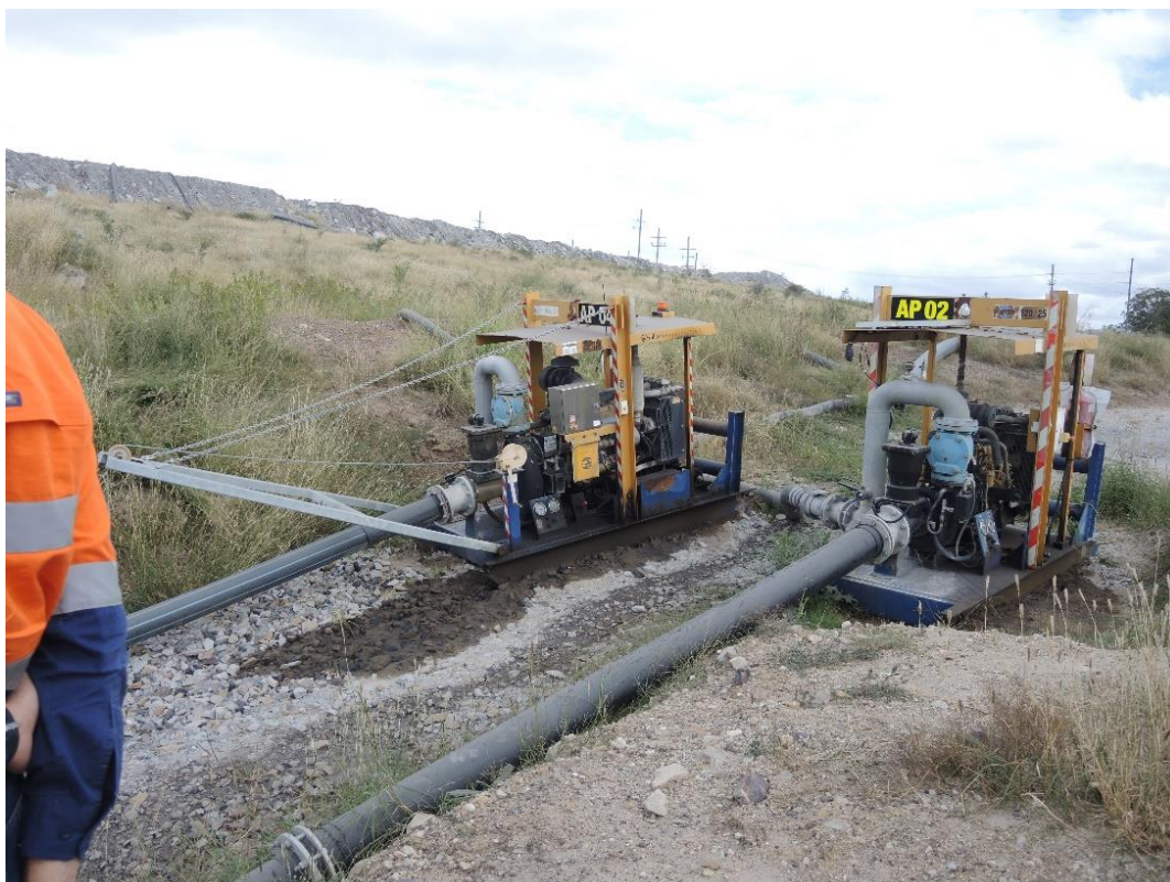
Plate 10 A second water pump installed at Dam46N in response to incident 30/3/19
