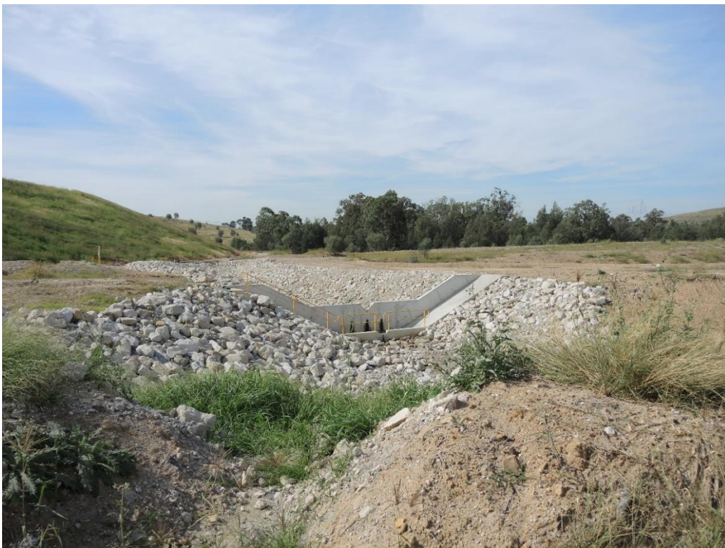
Plate 12 Newly constructed water management system south of Dam 9s
