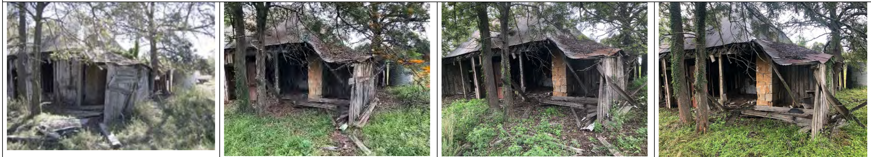
South-eastern corner 2014-8: vertical slabs have been removed causing further collapse of roof. 2018-20 (Mar): further deterioration of eastern wall. Mar 2020-Dec 2020: heavy leaf litter on roof persists.
