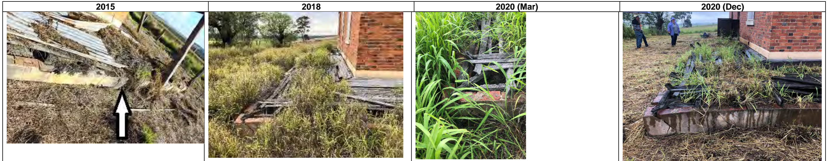
View of eastern verandah (focus on dwarf wall wall) 2015-8: debris cleared from verandah, no change to dwarf wall 2018-20 (Mar): no discernible change Mar 2020-Dec 2020: cracking to wall evident
