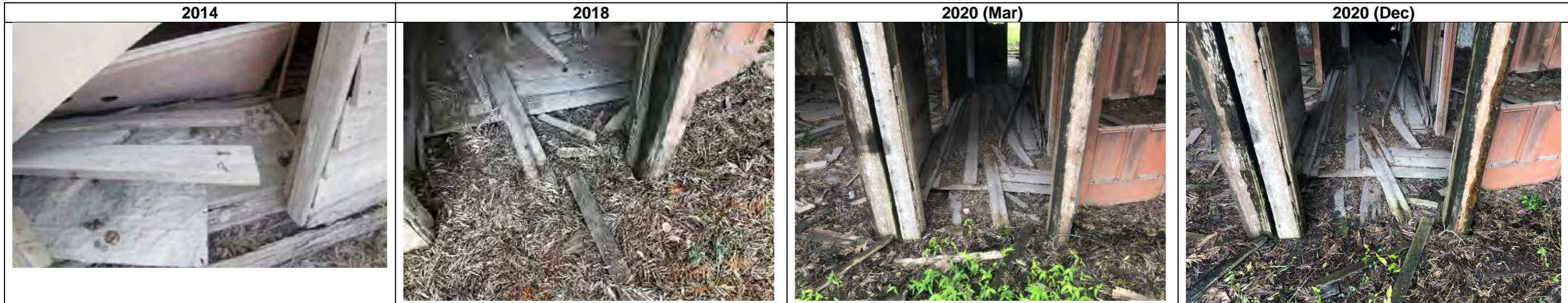
Southern elevation doorway 2014-8: door has been removed. 2018-20 (Mar): no discernible change. Mar 2020-Dec 2020: no discernible change.
