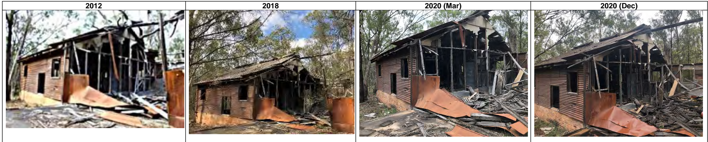
View to building interior from north-east 2012-18: shows collapse of remnant roofing members above open kitchen area. 2018-20 (Mar): further minor deterioration of asbestos sheeting panelling. Mar 2020 – Dec 2020: no discernible change.
