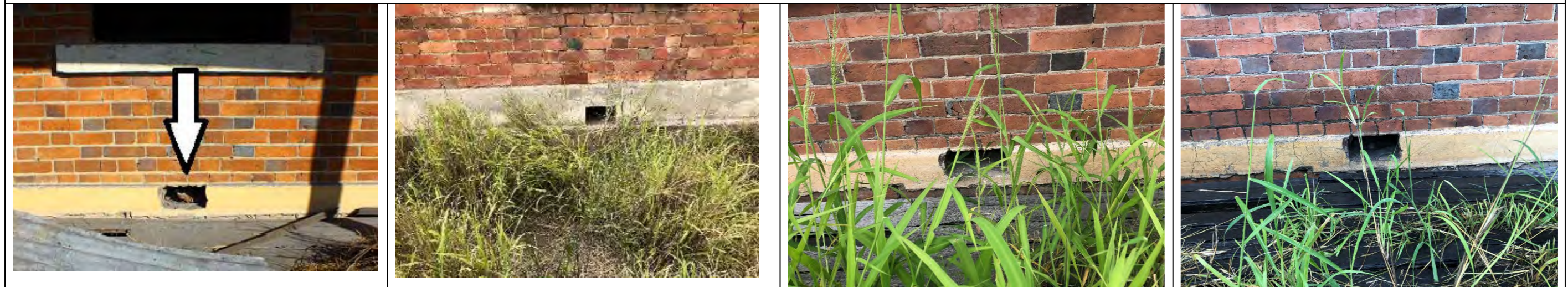
View of ventilation grilles 2015-8: grilles not replaced 2018-20 (Mar): no discernible change Mar 2020-Dec 2020: grilles remain open
