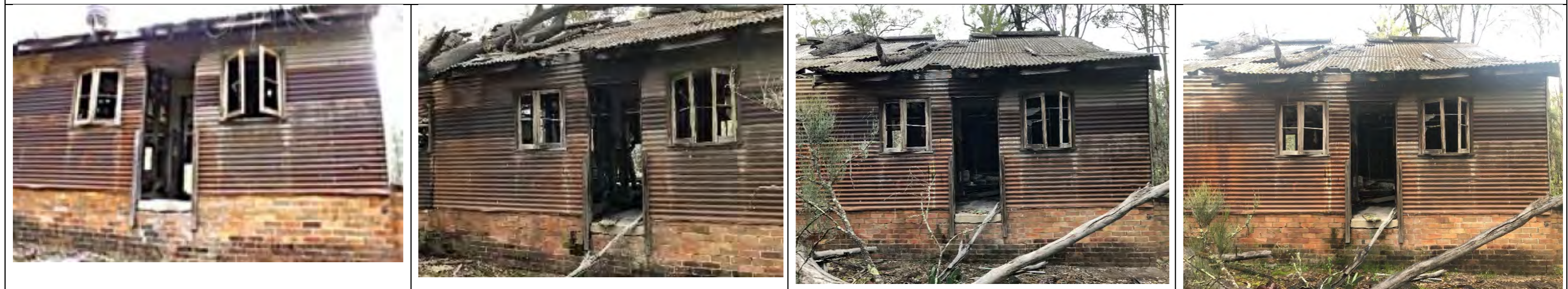
Windows and entry at west elevation 2012-18: shows large trunk/branch portions of tree collapsed on roof, which has destroyed roof ventilator. 2018-20 (Mar): shows majority of branches fallen from roof, leaving increased damage to sheeting. Mar 2020 – Dec 2020: no discernible change.
