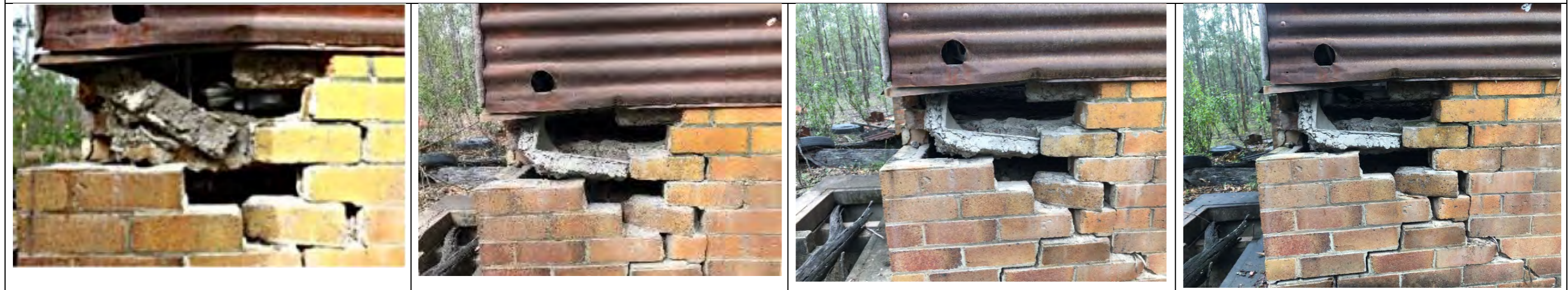
Detail of damaged brick foundation 2012-18: some further collapse of concrete/cement above brick foundation. 2018-20 (Mar): some slumping outwards of corner brick foundation. Mar 2020 – Dec 2020: no discernible change.
