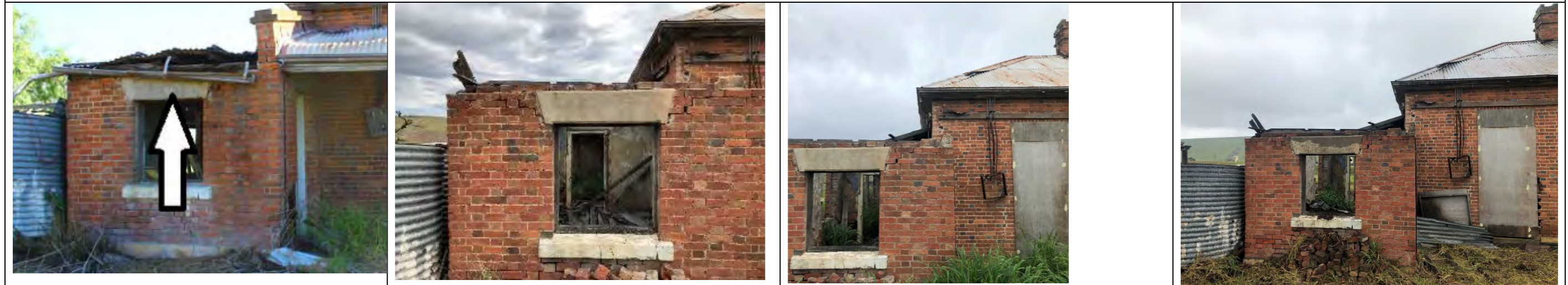
View of north-east of building 2015-8: wall element has collapsed (bricks stacked under window); roof framing, sheeting and guttering has collapsed 2018-20 (Mar): no discernible change Mar 2020-Dec 2020: no discernible change
