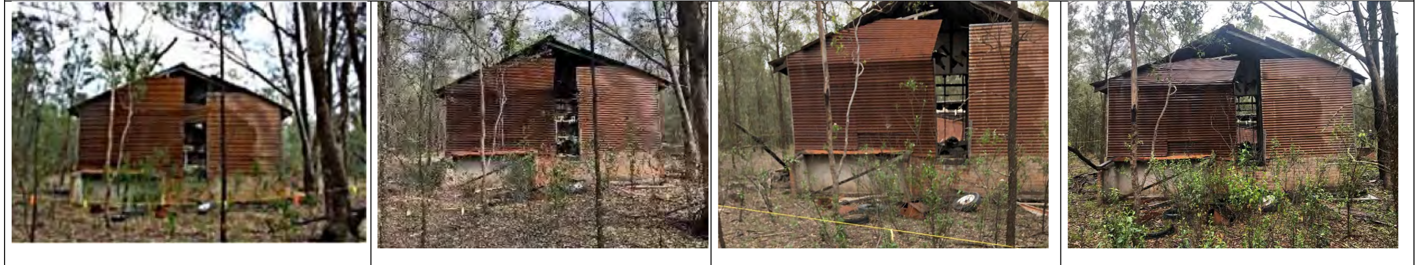
South elevation 2012-18: evidence of increased bow to southern wall and missing panel above entry. 2018-20 (Mar): increased bow to southern wall. Mar 2020 – Dec 2020: increased bowing on southern wall.
