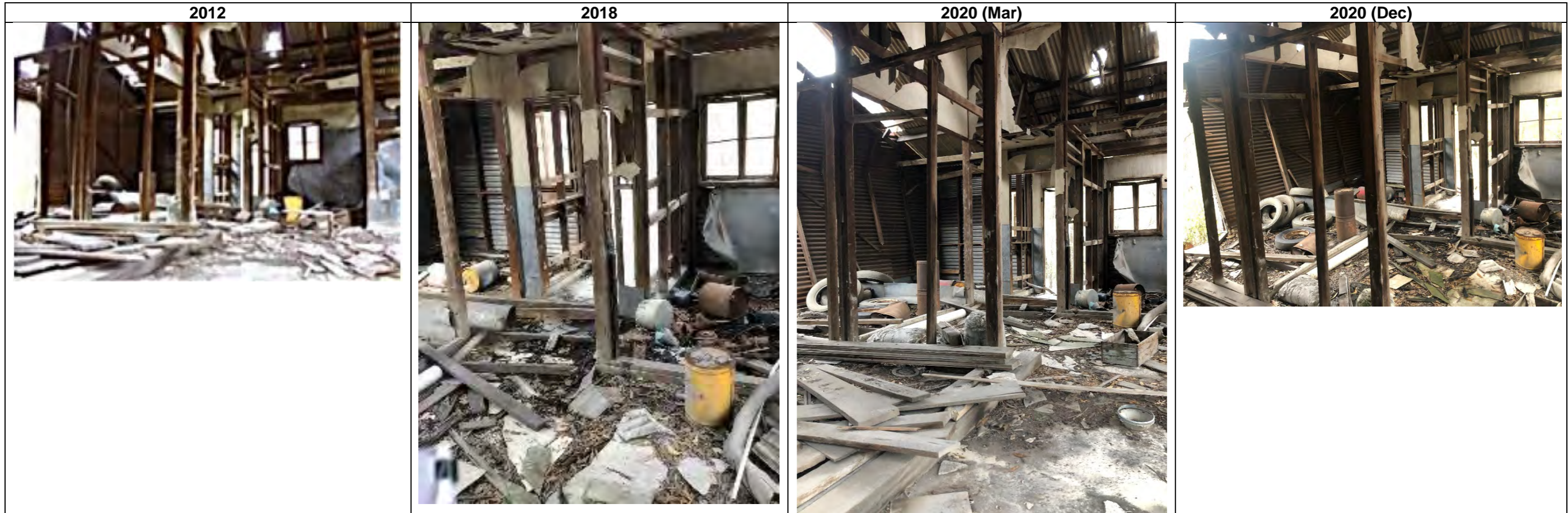
View to interior, showing west entry to building 2012-18: no discernible change. 2018-20 (Mar): no discernible change. Mar 2020 – Dec 2020: no discernible change.
