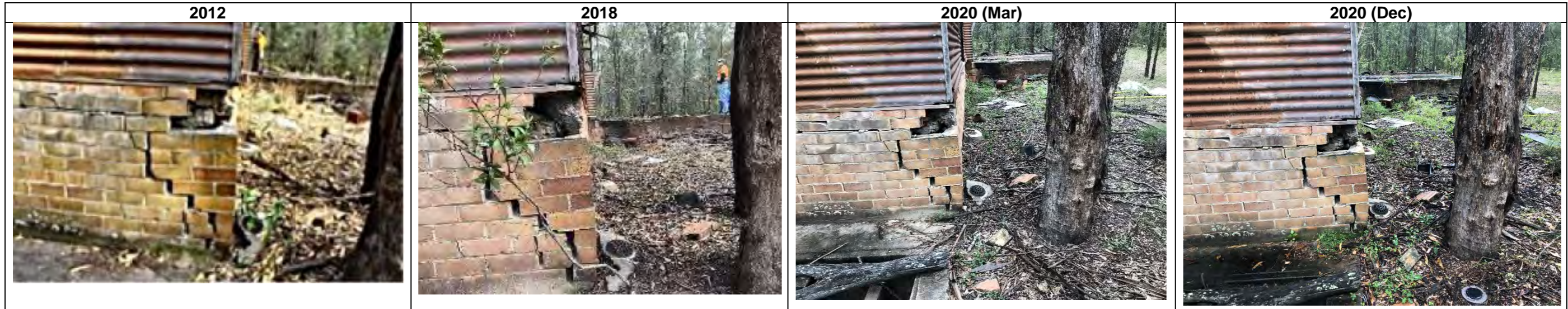
Damaged brick foundation at south-east corner 2012-18: no discernible increase to cracked brick foundation. 2018-20 (Mar): further cracking of foundation (to left of shot) and some slumping of corner bricks. Mar 2020 – Dec 2020: some slight potential further movement in cracked section (also note termite management system in bottom right hand corner of photograph).
