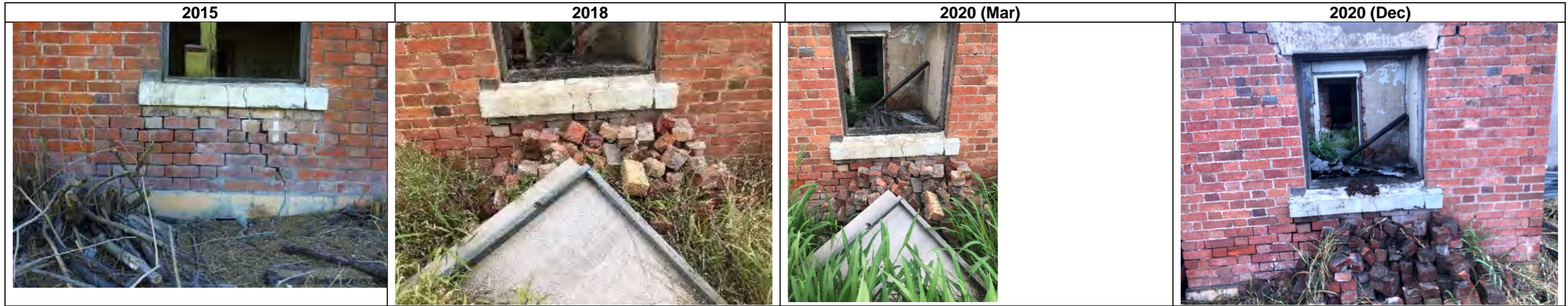
View of north-east corner of building (focus wall below window) 2015-8: bricks from roof above stacked in front of required repointing, window sheeting removed 2018-20 (Mar): no discernible change Mar 2020-Dec 2020: repointing requirements remain
