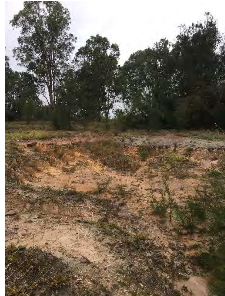
Plate 37 Erosion (top of right bank)
