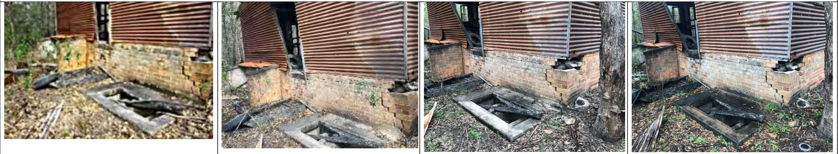
Grease trap at south end of building 2012-18: shows bow to south wall. 2018-20 (Mar): shows increased bow to south wall. Mar 2020 – Dec 2020: shows increasing bowing of south wall, and example of new termite monitoring system in bottom right of picture.
