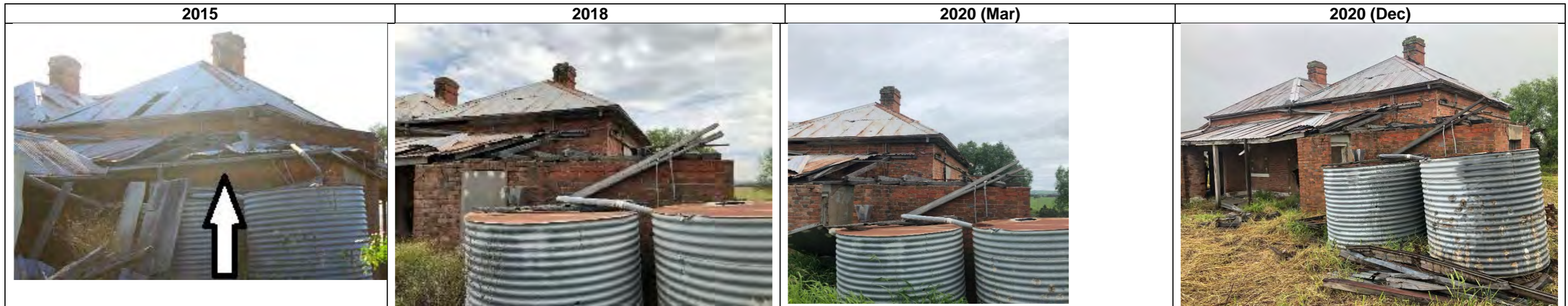
View of rear of building (focus on roof) 2015-8: skillion roof, guttering and rafters have collapsed; main roof holes repaired 2018-20 (Mar): no discernible change Mar 2020-Dec 2020: some minor holes in roofing require repair
