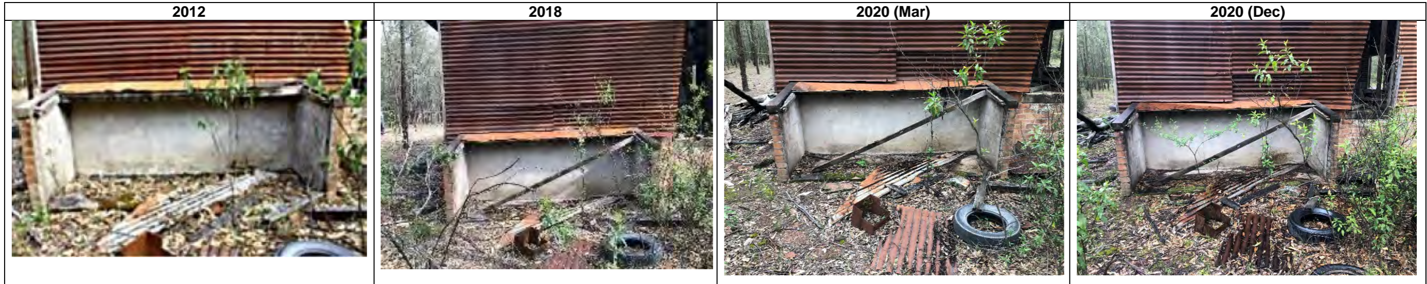
Storage area at south end of building 2012-18: further slight collapse of storage area. 2018-20 (Mar): shows loosening of corrugated iron wall sheeting due to bowing in wall. Mar 2020 – Dec 2020: no discernible change.
