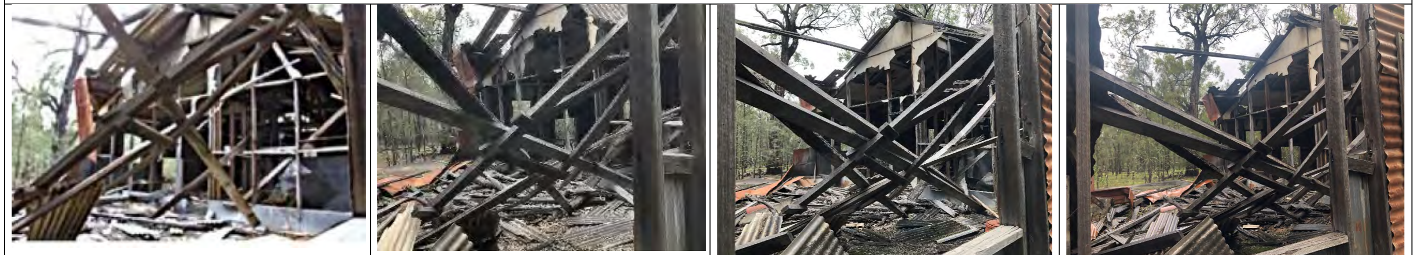
Showing interior of building, viewed from north-west corner 2012-18: shows collapsed roofing members above open kitchen area and accumulation of debris. 2018-20 (Mar): shows additional collapsed roofing member. Mar 2020 – Dec 2020: no discernible change.
