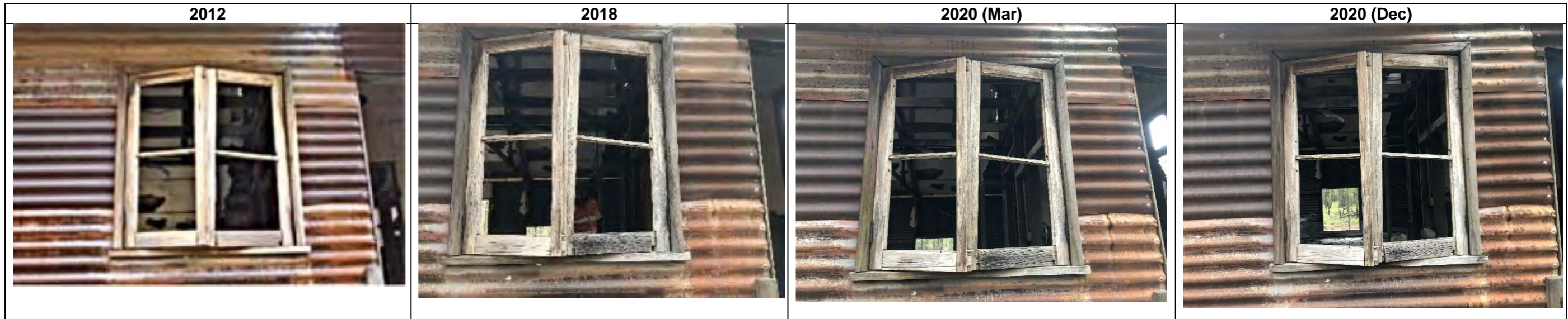
Timber window detail, west elevation 2012-18: no discernible change. 2018-20 (Mar): no discernible change. Mar 2020 – Dec 2020: no discernible change.
