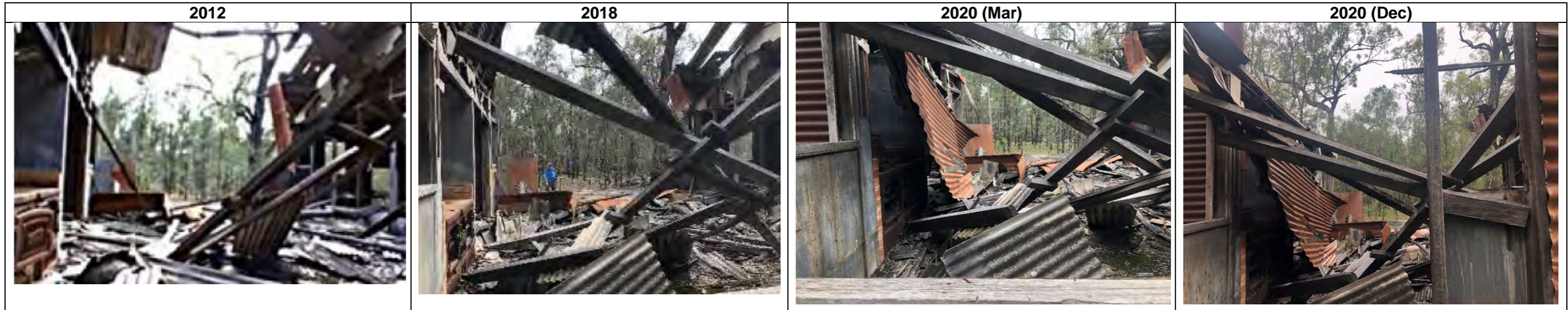
Showing interior of building, viewed from north-west corner 2012-18: shows collapsed roofing members above open kitchen area and accumulation of debris. 2018-20 (Mar): shows collapsed north wall across stove and additional fallen roof member. Mar 2020 – Dec 2020: no discernible change.
