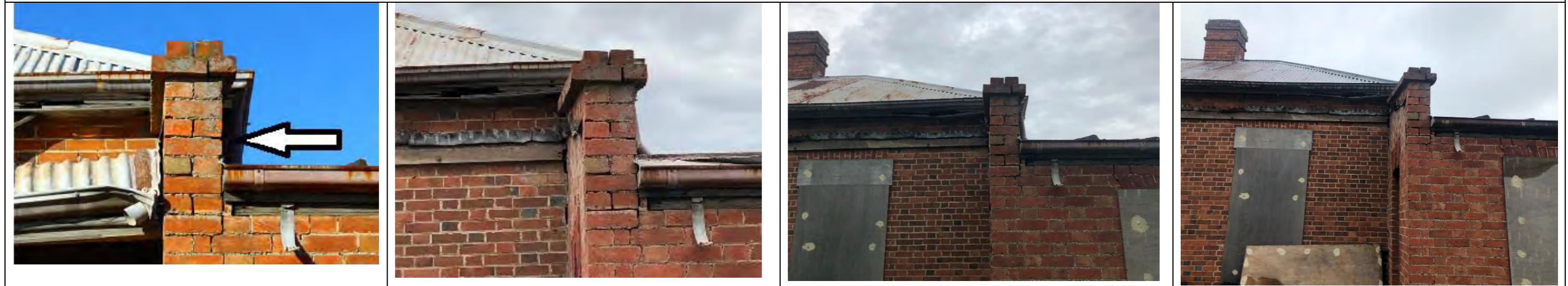
View of south-east of building (focus on top of wall) 2015-8: no discernible change 2018-20 (Mar): no discernible change Mar 2020-Dec 2020: no discernible change
