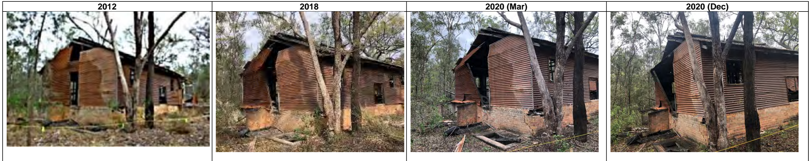
South-east elevation 2012-18: evidence of increased bow to southern wall. 2018-20 (Mar): bow in wall appears to have increased. Mar 2020 – Dec 2020: bow in wall continues to increase.
